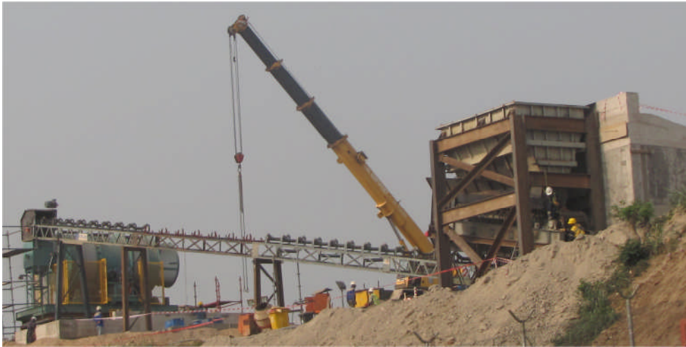
Newly designed CP plant
