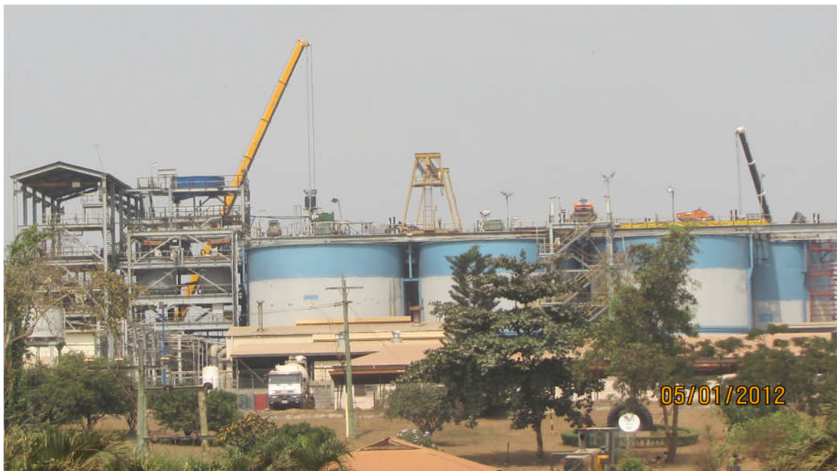
Refurbished CIL tanks
