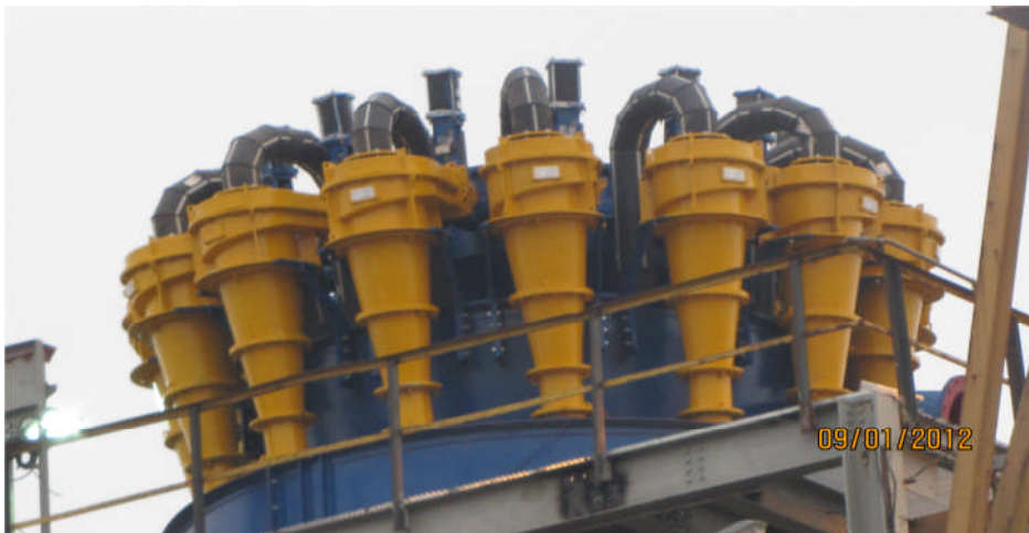
Cyclone Cluster ready to receive feed from the Ball Mill circuit
